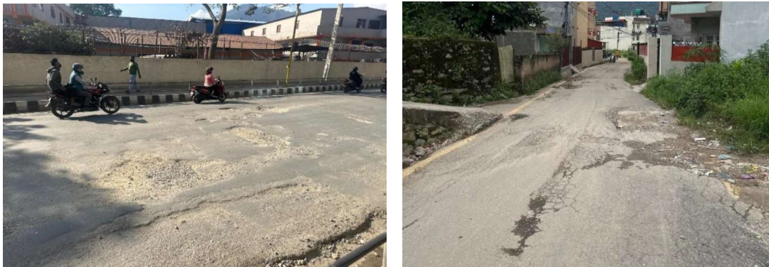
Figure 1.1 Pavement Failure Observed In Road Network Within KMC
