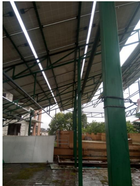
Figure 4-9: Roof-mounted solar panel in Saligram Hotel
