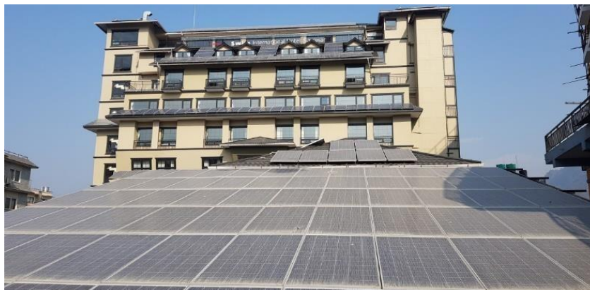
Figure 4-8: Solar panels on roof
