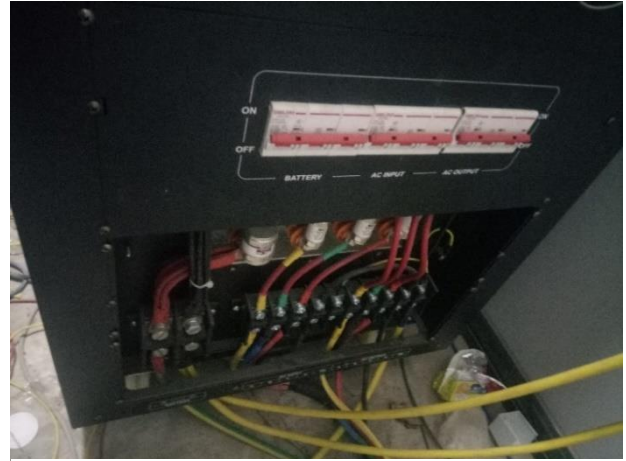
Figure 4-5: Low frequency three phase solar Inverter (50KVA)
