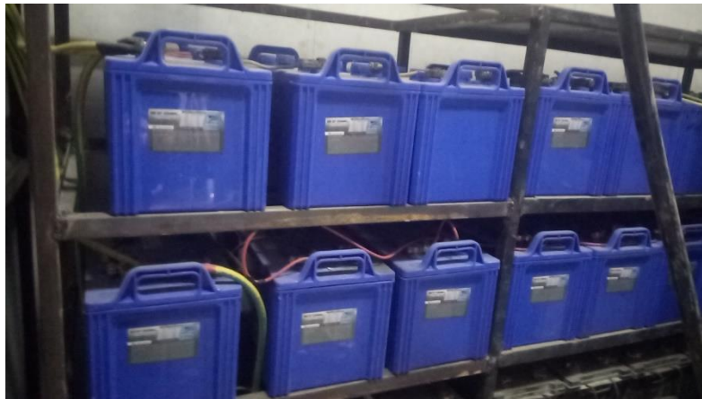
Figure 4-6: Lead-acid Batteries used for the energy storage
