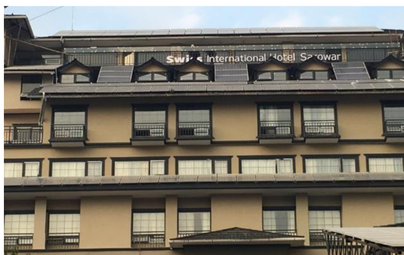
Figure 4-9: Solar panels on roof
