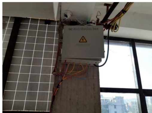
Figure 4-2: Solar- DC Distribution Box in the first floor
