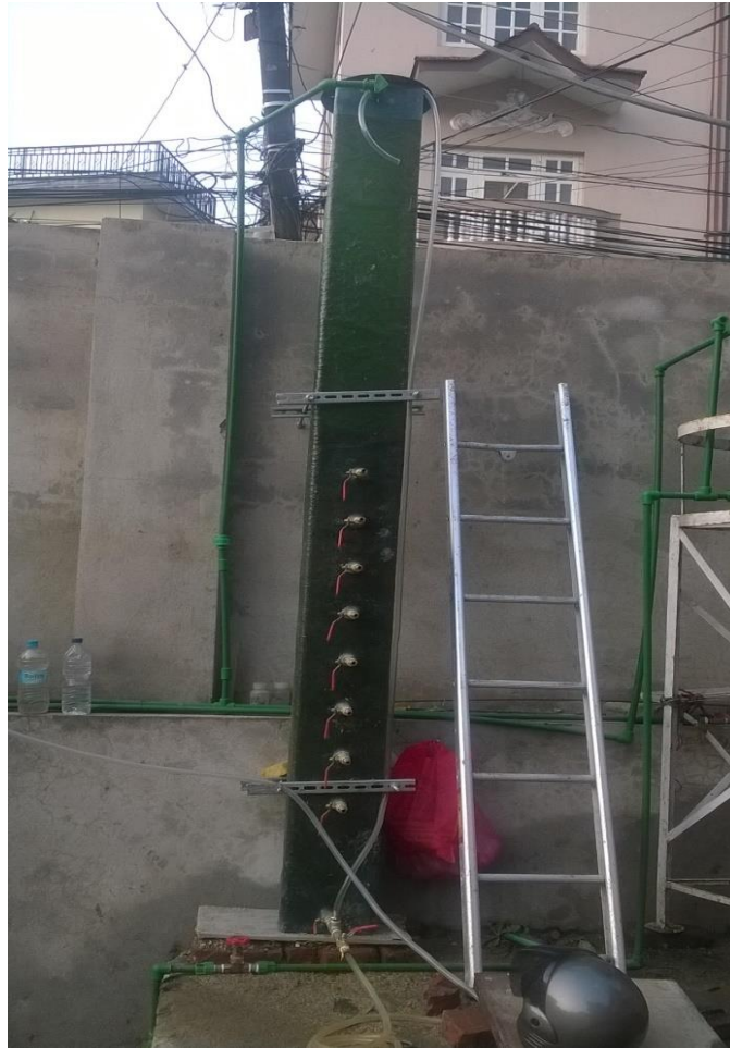
E.3 Filter setup installed at ECD, IOE
