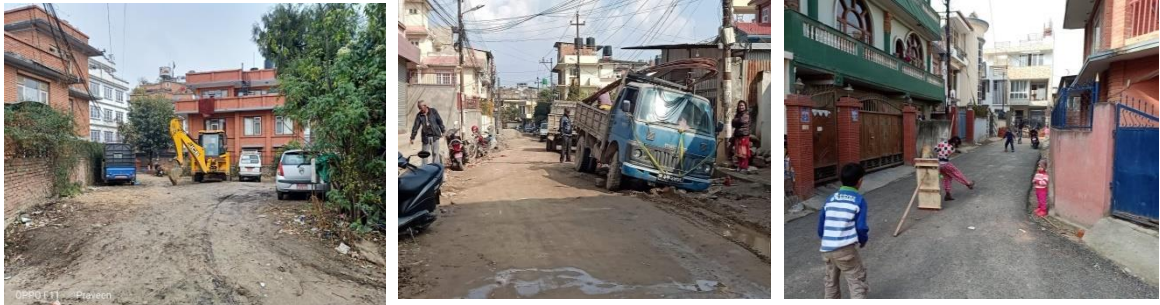
Figure 30 Streets (Installation of Melamchi water pipeline, Truck stuck on road, Children playing in Inner Street)
