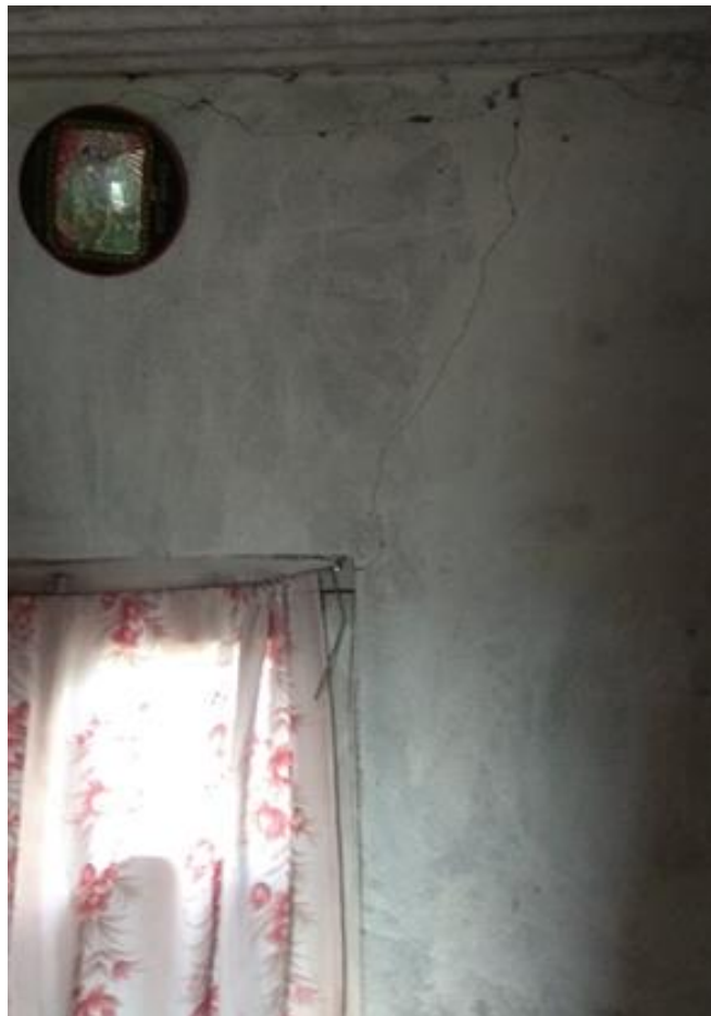
Fig: Diagonal cracks from opening
