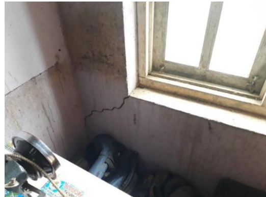
(b) Diagonal Cracks originating from opening
