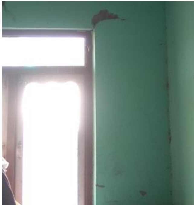
Figure: Diagonal cracks from opening
