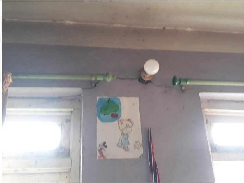
Fig: Cracks through pier
