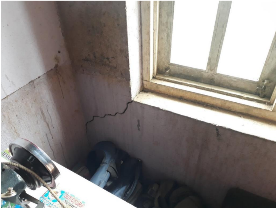
Figure: Diagonal cracks from opening
