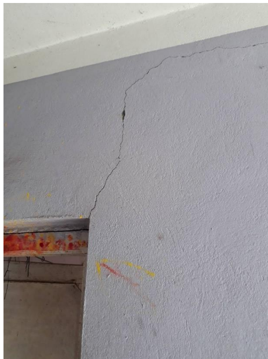
Fig: Cracks from opening
