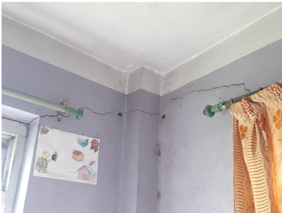
Fig: Cracks from opening to opening
