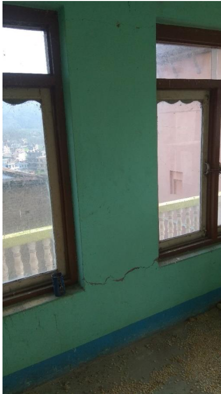
Figure: Cracks through pier
