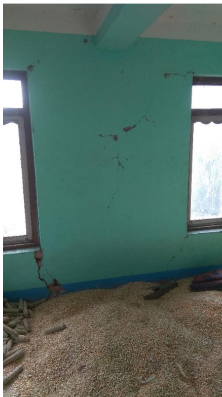
Figure: Diagonal cracks from opening
