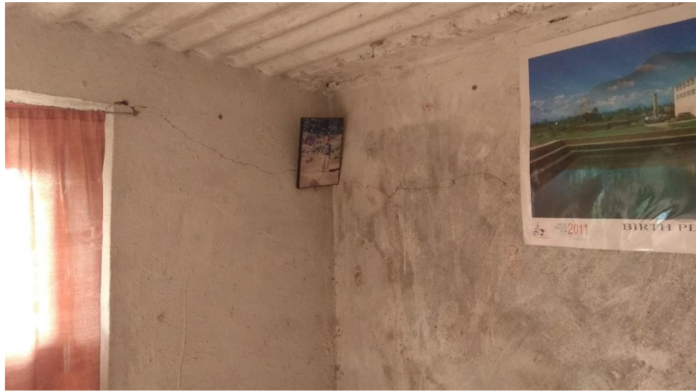
Fig: Cracks from opening
