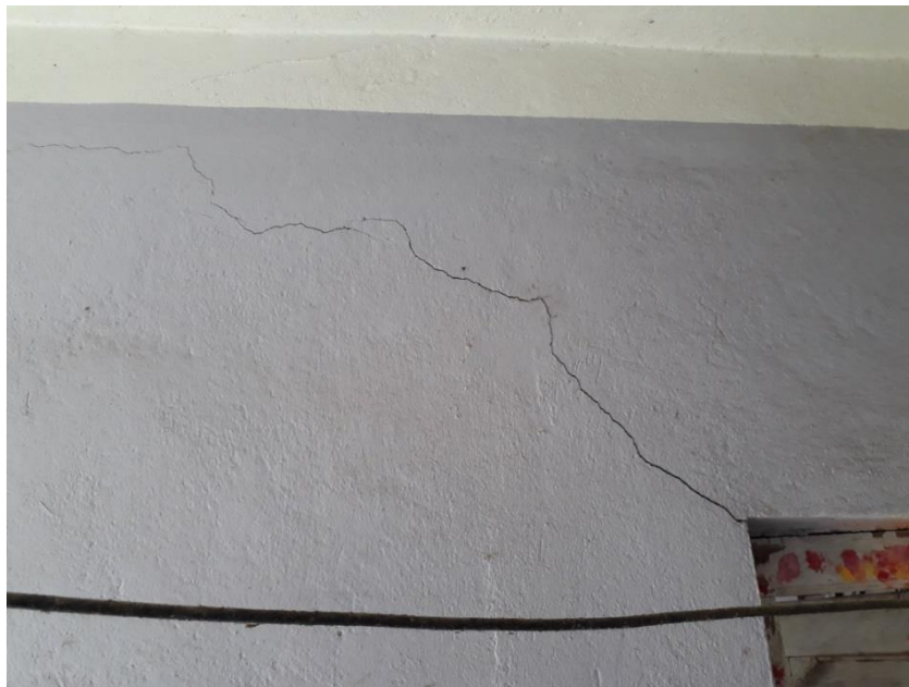
Figure: Diagonal cracks from opening
