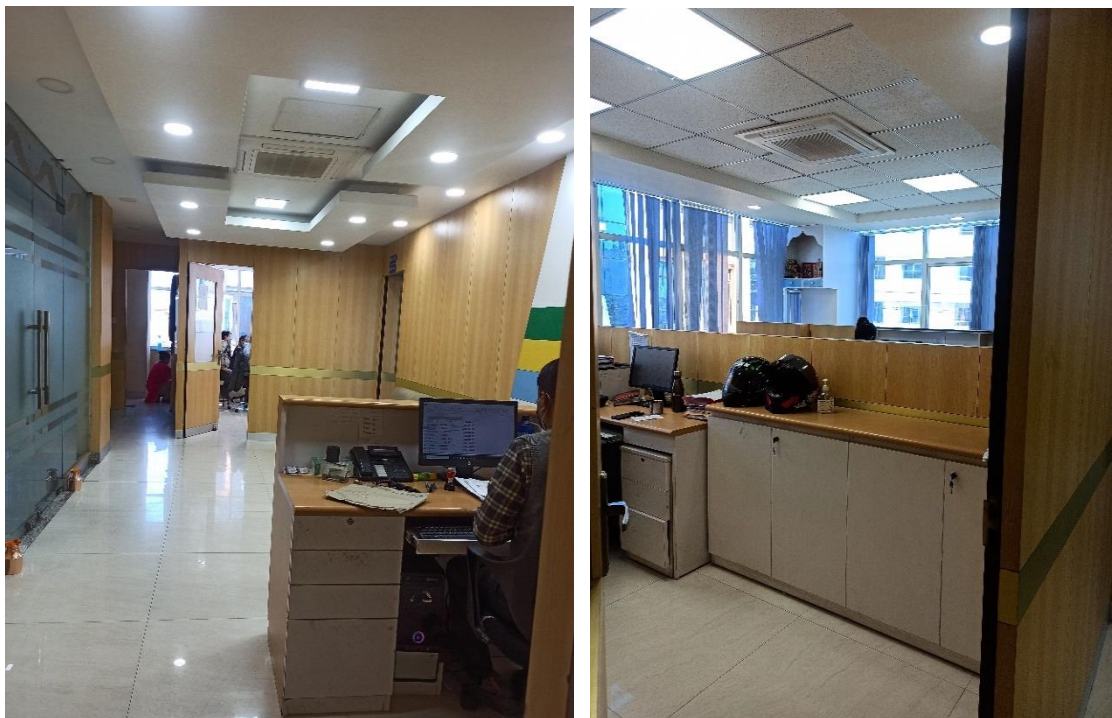
Figure 37: Showing Lighting at Reception and Working Spaces
