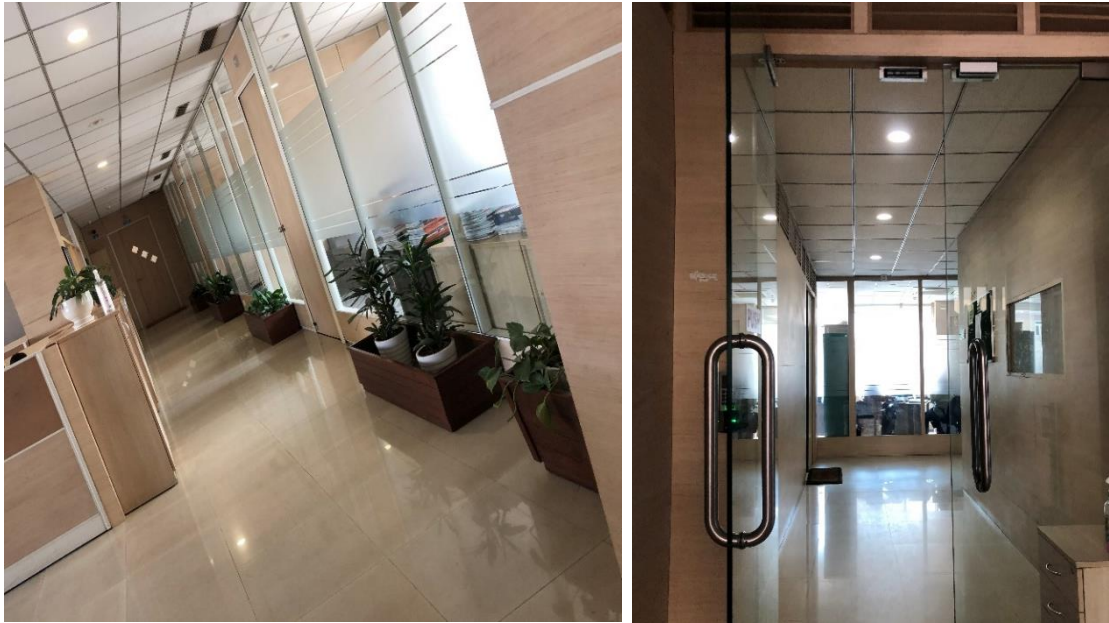
Figure 59: Internal Lighting in Passage-BPC
