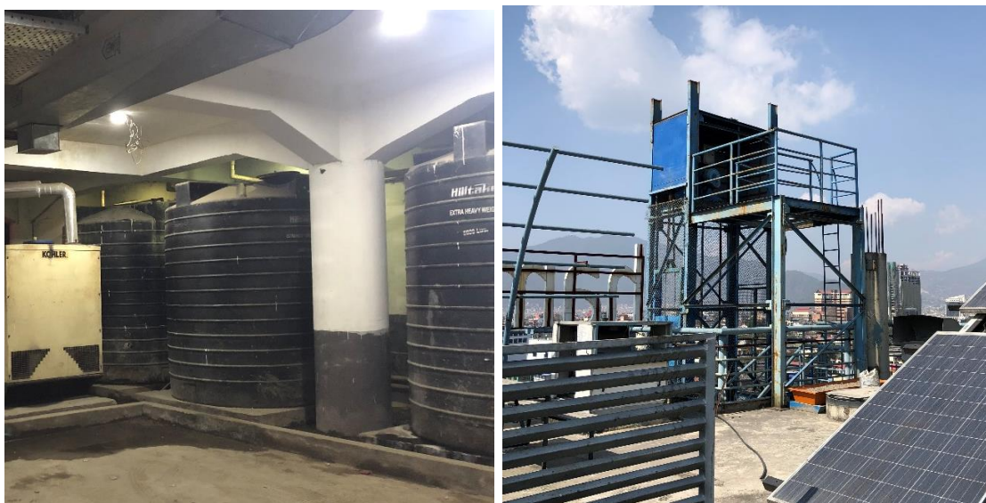
Figure 40: Storage for Rain Water and Separate Service Lift at West
