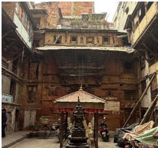
Figure 81: Harsha Chaitya Vihar in dilapidated condition in Haku Baha
