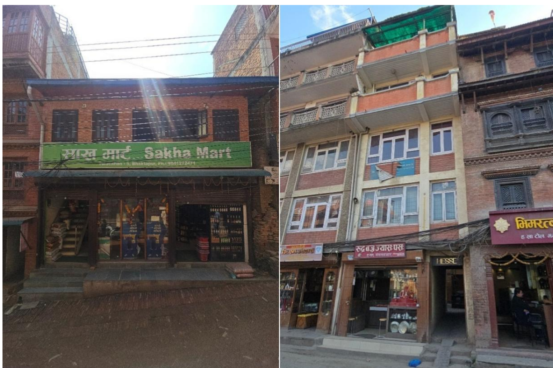
Picture 6 Examples of Non-compliance (flat rooftop violations)
