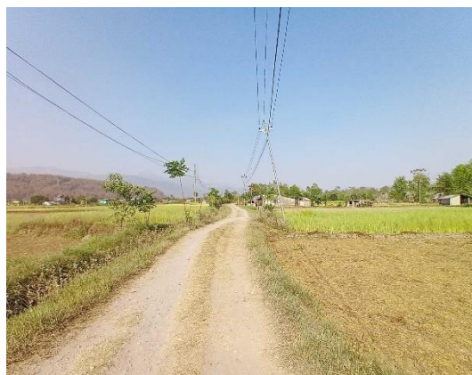
Condition of Road in Ward No. 2
