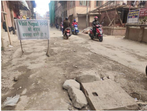
Figure 5: Figure showing the damaged road condition in Saugal road.
