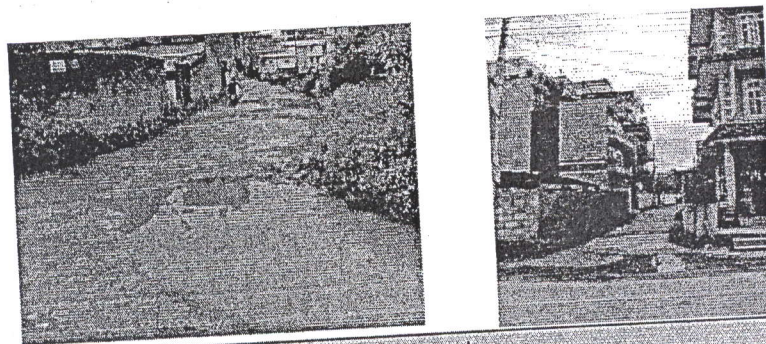
Figure 49: Water logging in the roads
