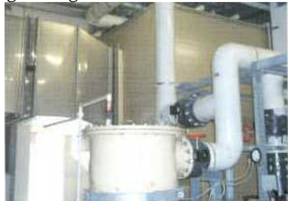
Figure 108: Water scrubber to reduce odours
