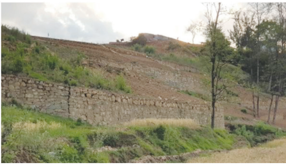
Branch canal requiring maintenance
