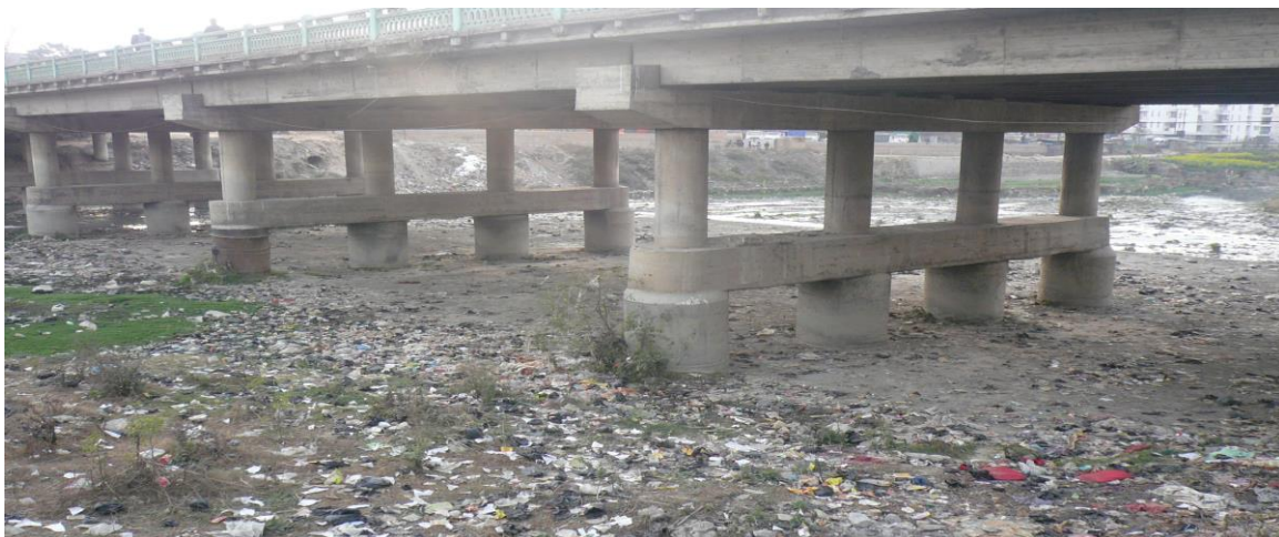
Fig. 1.3 Balkumari Bridge at Koteshawar (Pile cap is completely exposed above the bed level. Pile is exposed above 1.6m from the bed level)
