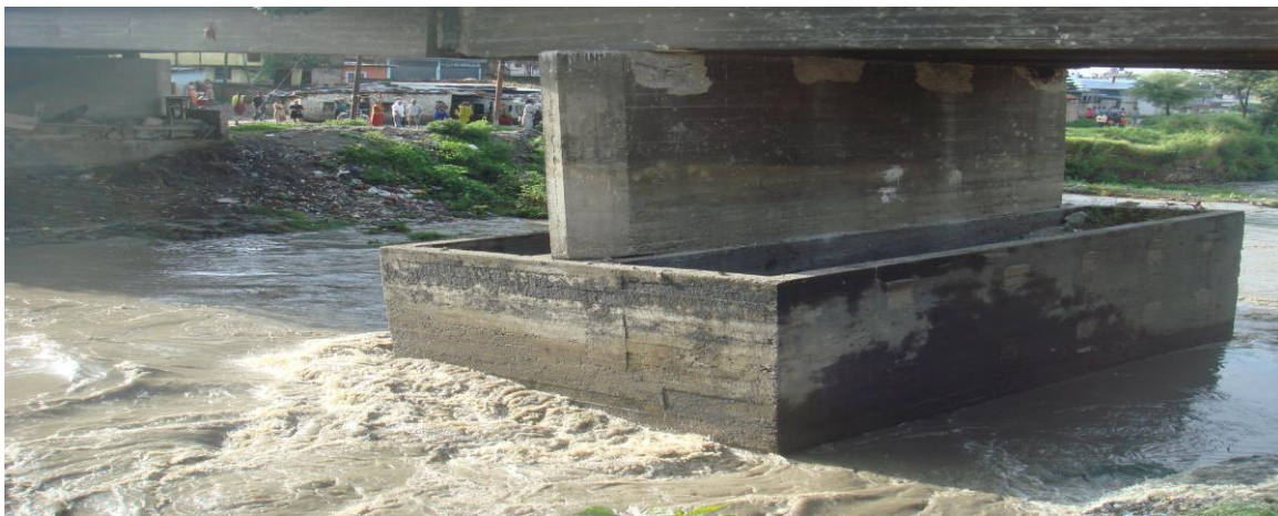
Fig. 1.2 Sinamangle Bridge (scouring; exposure of pier cap)
