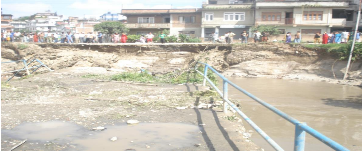
Fig. 1.1 Sinamangle Bridge (The Bridge collapsed and fell below the road level).
