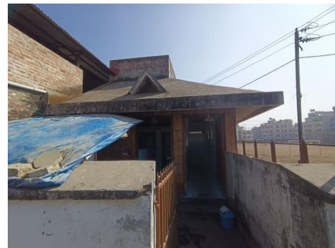
Figure 18 Public toilet with no signage and indications
