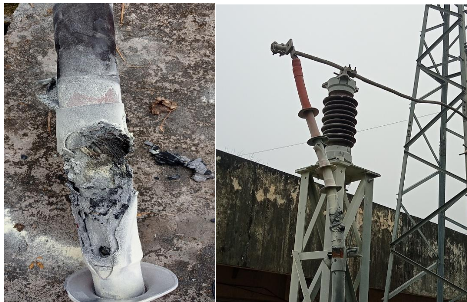
Figure 4.7 33 kV UG cable termination damaged
