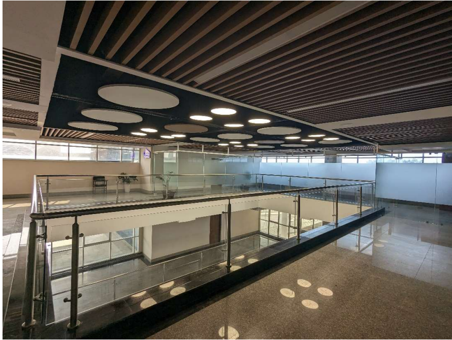
Figure 44: Internal Lighting Fixtures
