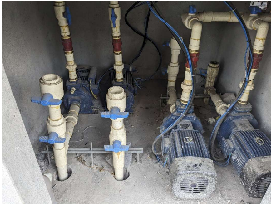
Figure 41: Pumps installed for lifting water
