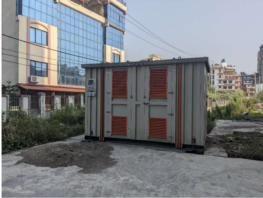
Figure 38:630KVA CSS(Compact Substation)
