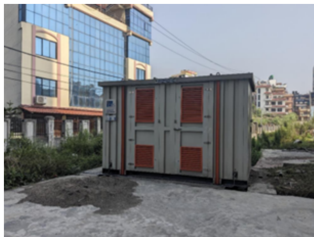
Figure 3: 630 KVA Compact Substation installed on site
