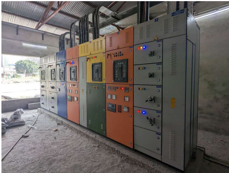
Figure 39:LT Panel installed on site (incoming from CSS to raising mains)
