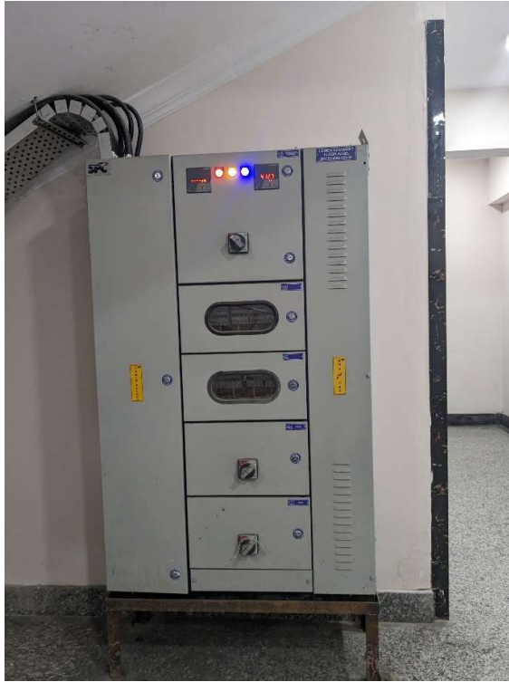
Figure 40: Raising mains/Floor panels (incoming from LT Pannel and Feed to DB)
