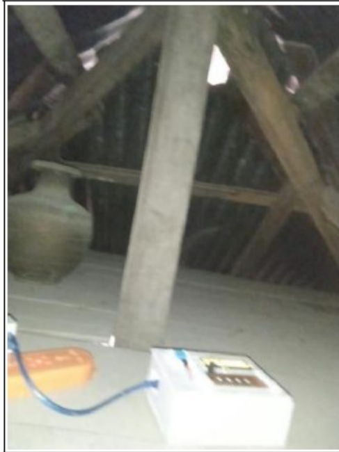
Figure 9: Datalogger placed inside Attic space
