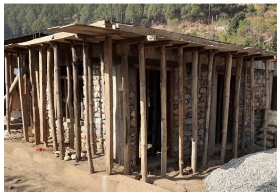
Figure 17 RCC building with stone cement wall under construction post disaster in Rimna
