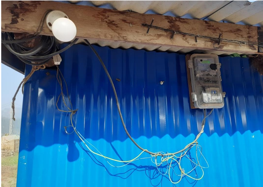
Figure 25 Electric meter in temporary shelter
