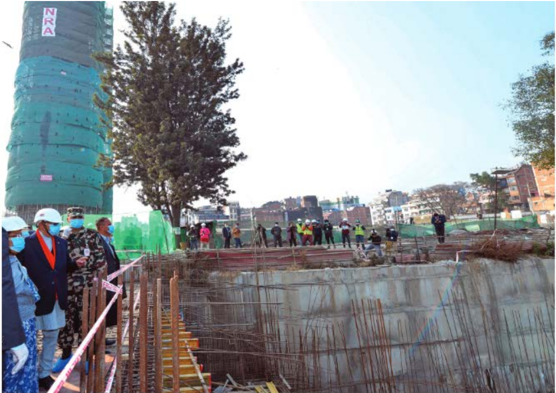
Prime Minister KP Sharma Oli inspecting work progress in Dharahara reconstruction in Kathmandu on Thursday.
