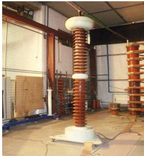
Figure 2. 9: Load capacitor and its external resistor AUTH laboratory
