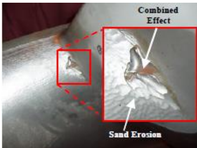
Figure 2. 15 Eroded part of Turbine Runner with pure sand erosion and combine effect demarcated (Upadhyay, 2007)
