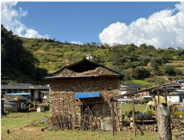
Partially destroyed house in Barekot 1
