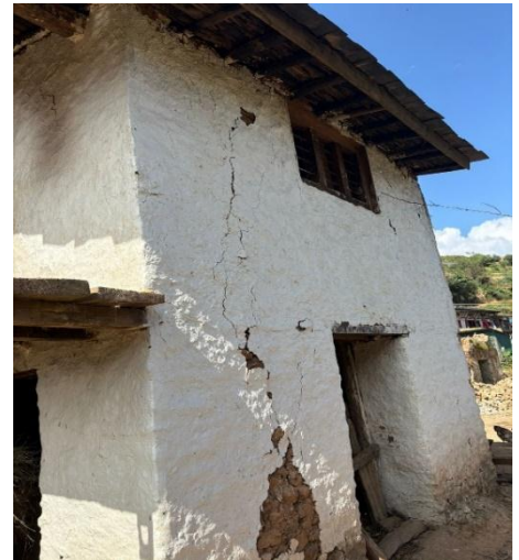
Partially destroyed house in Barekot 3
