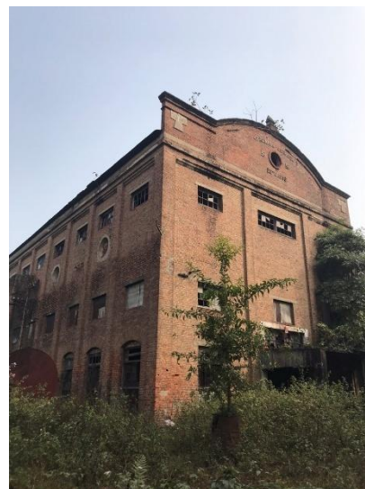
Figure 29 Turbine House BJM
