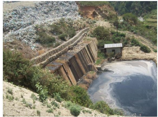
Figure 36: Leachate flow from the landfill to the river
