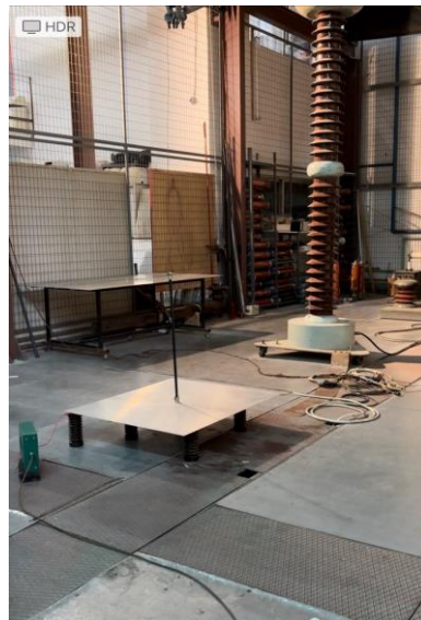
Figure 3.17: Test transformer connection-grounding
