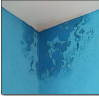
Figure: Seepage inside rooms due to poor construction quality
