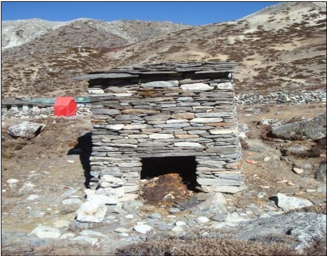
b) Public toilet at Chukkung. Toilet waste flows out on the surface near the water course.
