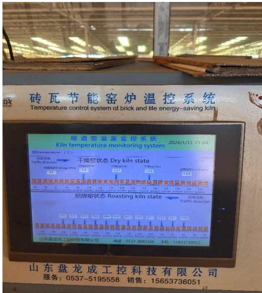
Kiln Temperature Monitoring system
