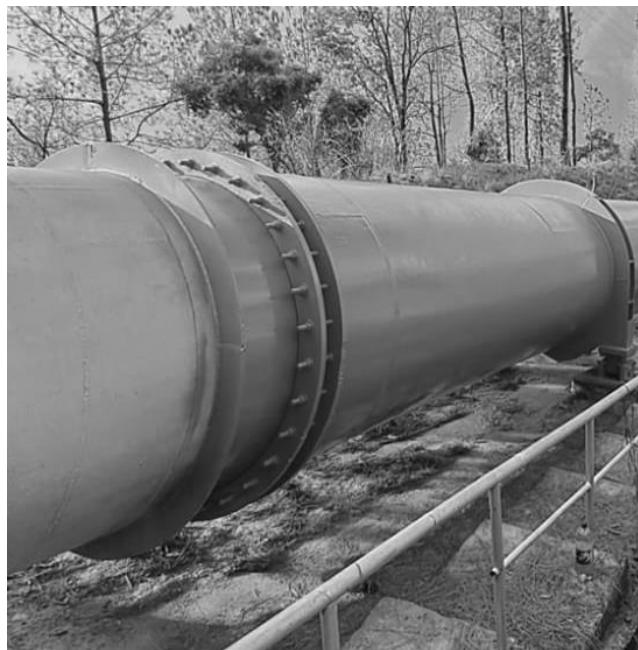
Figure 2. 2: Penstock with Expansion Joint
