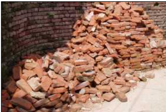
Low quality bricks in use
