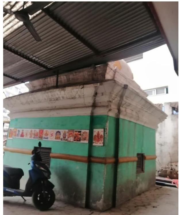
Figure 25: Iron rod piercing the roof of laxmisor Mahadev Temple
