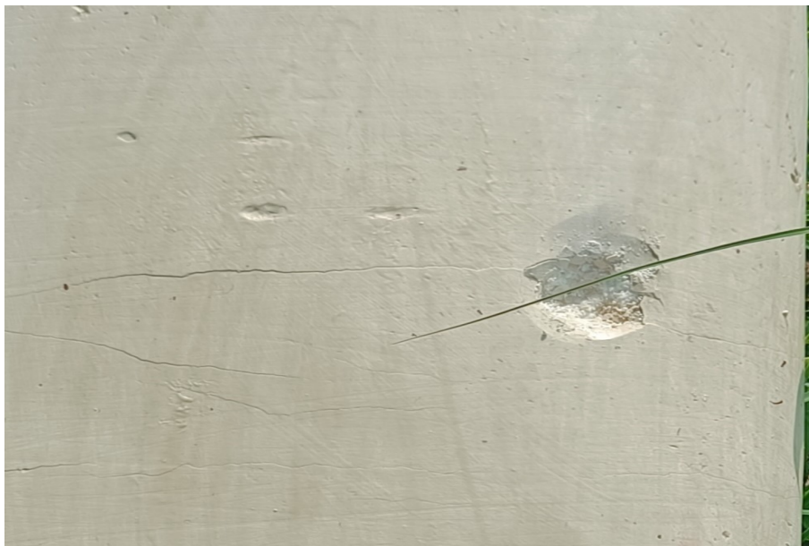
Figure 4.1: Foam molding failure
