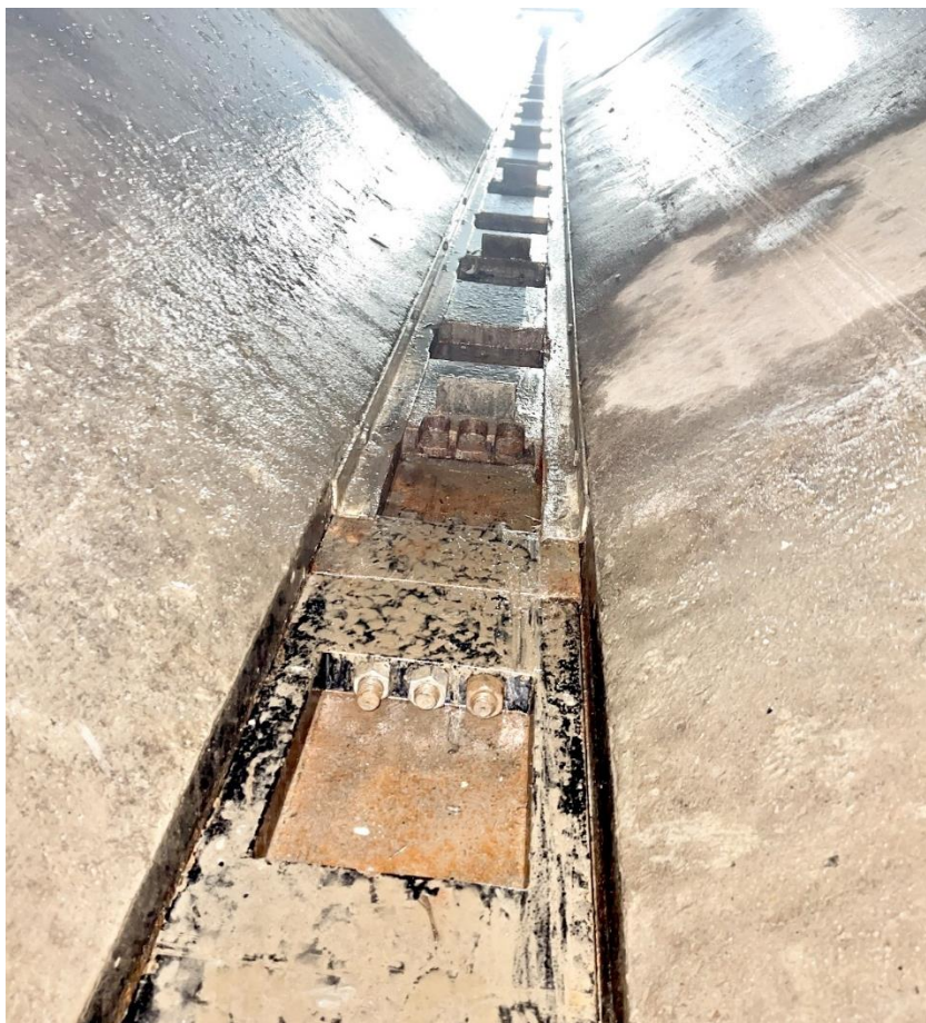
Figure 9 Bieri Vertical Sand Flushing System of MMHPP
