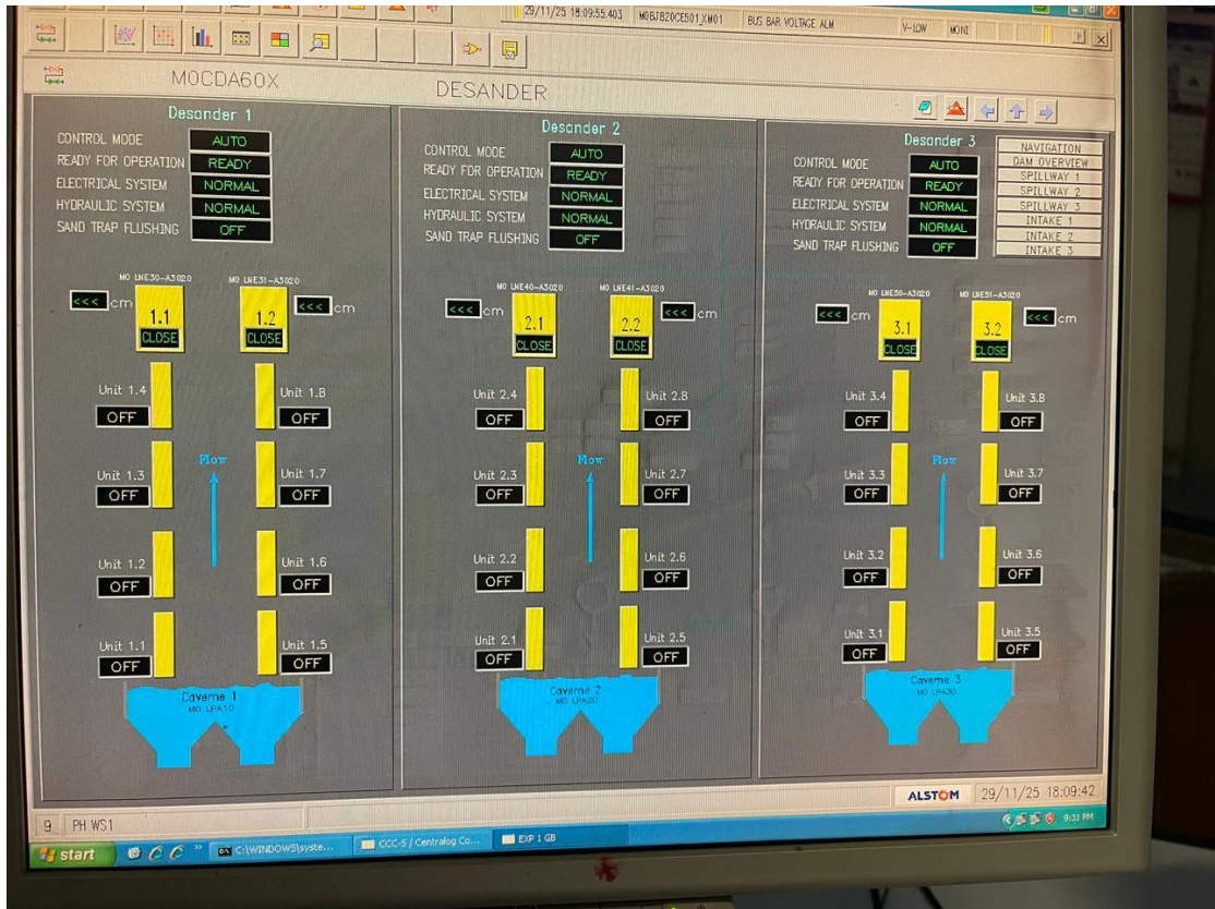
Figure 15 SCADA Layout of three Desander Units of MMHPP
