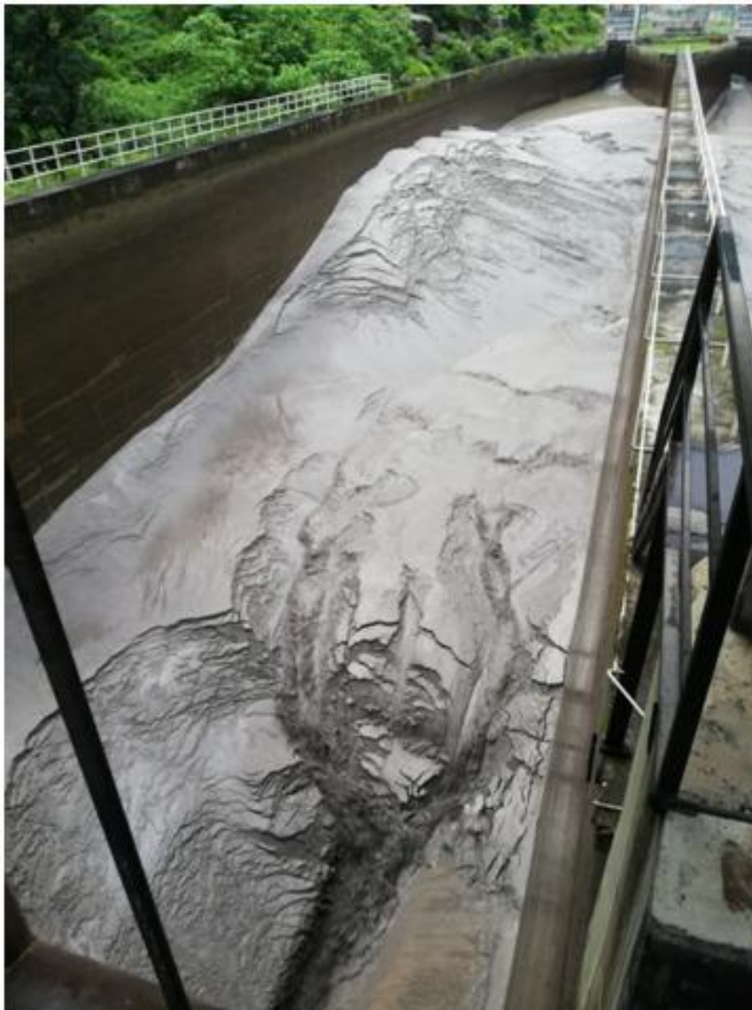
Figure 7 Sand Deposition at Desander of Upper Trishuli 3A HPP
