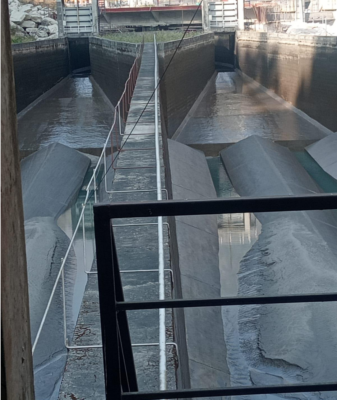
Figure 5 Desander(CSFS) of UT3A HPP
