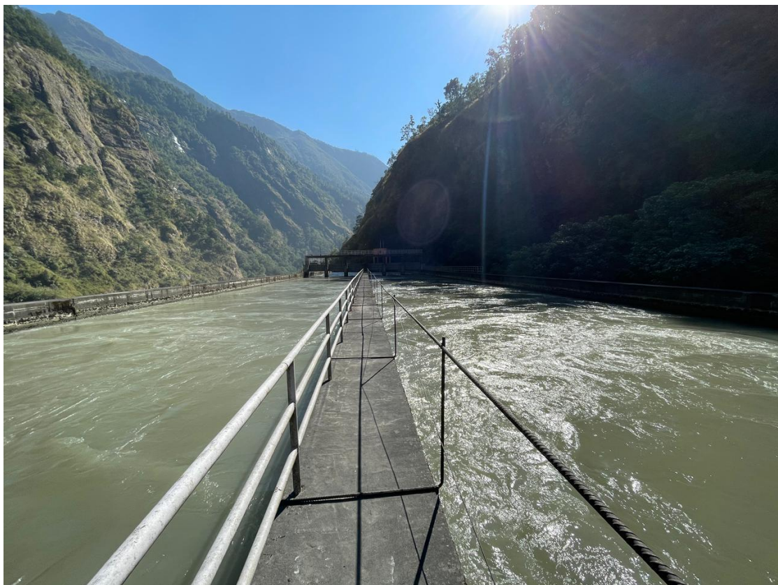
Figure 16 Two Desander units of UT3A HPP
