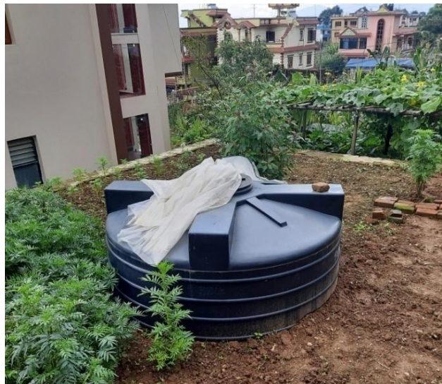
Rainwater Collection Tank in Kirtipur
