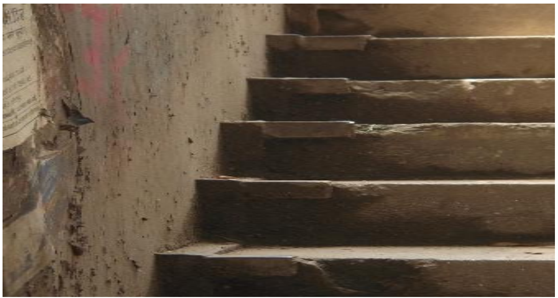
Figure 4.7 Bhotahity Bridge: Broken Edges of the Foot Steps
