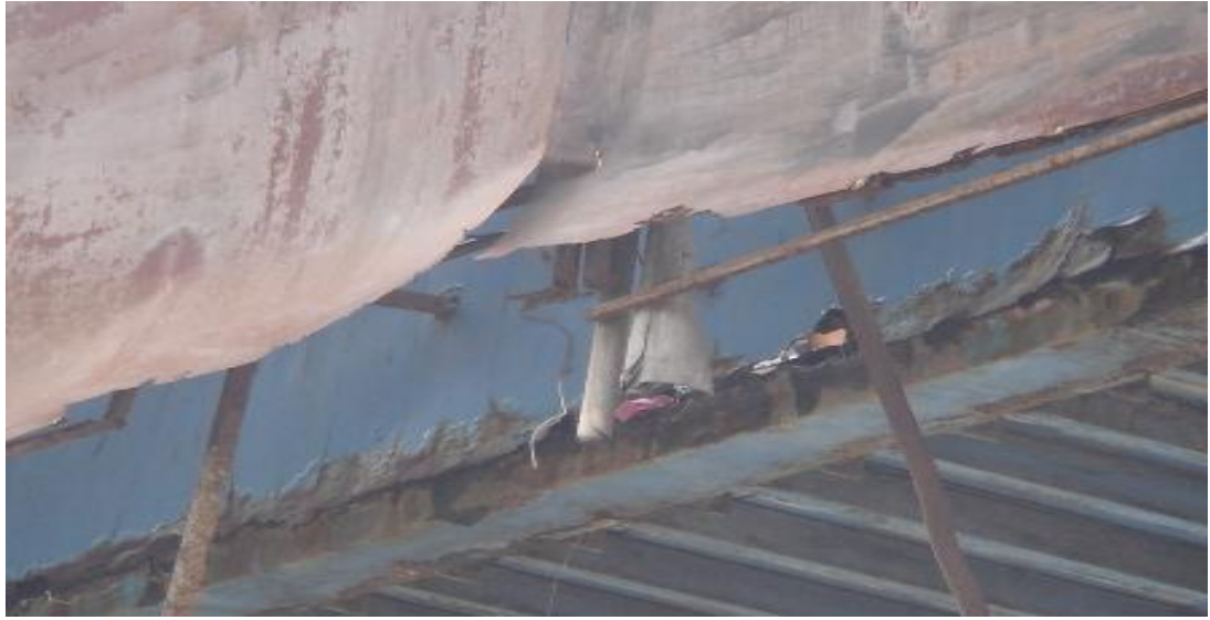
Figure 4.6 Bhotahity Bridge: In need of maintenance
