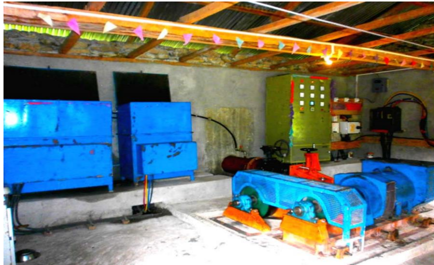
Figure 37: Electromechanical Equipments of Chimal MHP (District Development Committee, Taplejung, 2016)
