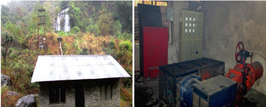
Figure 32: Power House (Left) and EM Equipments (Right) of Phawa Khola MHP (District Development Committee, Taplejung, 2016)
