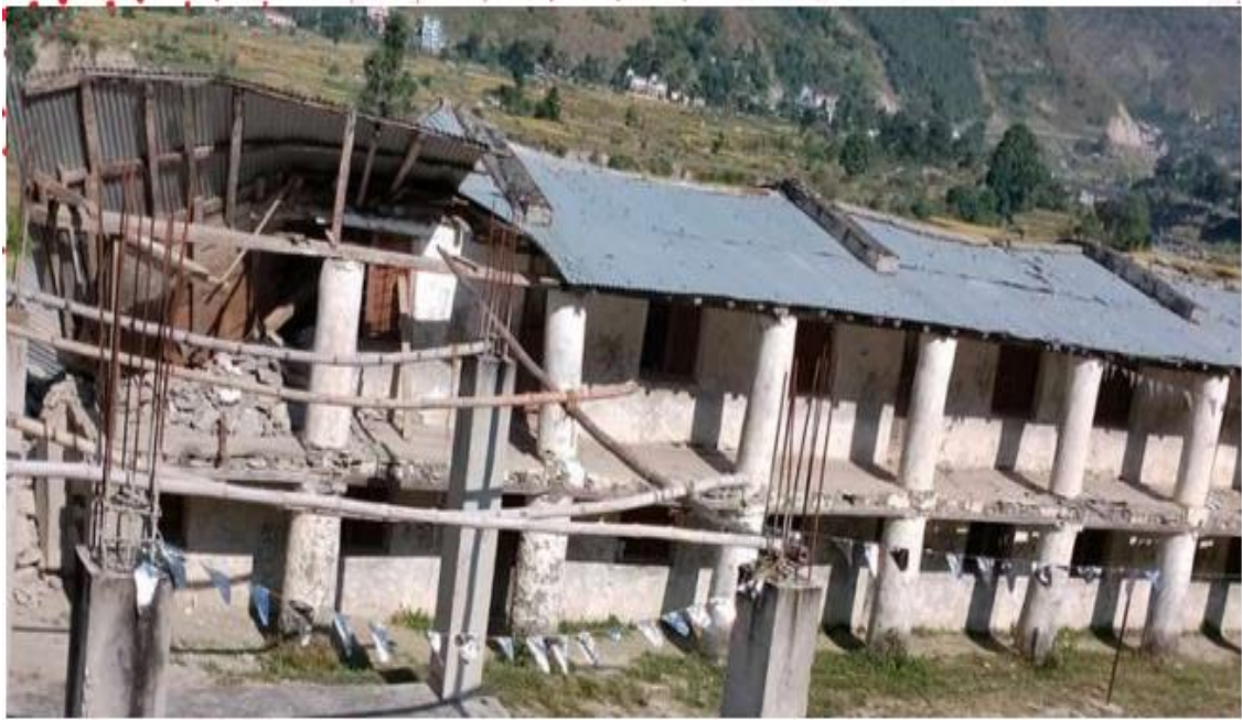
Balbikash School, Golae, Municipality after Earthquake
