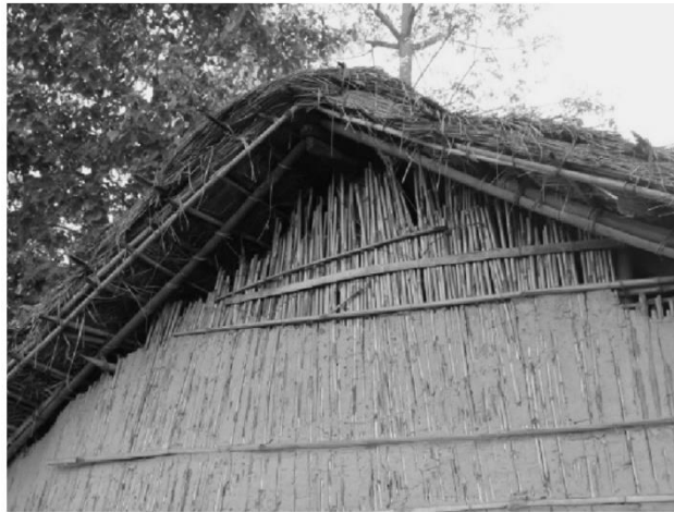
Figure 3: Gable opening for air circulation in Tharu House, Chitwan (Source: Bodach et. al.)
