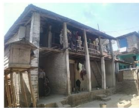
Fig: Addition of pillar and concrete block in old mud structure; Residence of Mr. Raj Kumar Chaudhary (School teacher)
