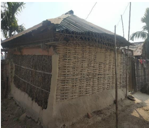
Figure 35: Combination of bamboo strips in one wall and straws, bamboo leaves and nigalo bamboo with mud on another wall
