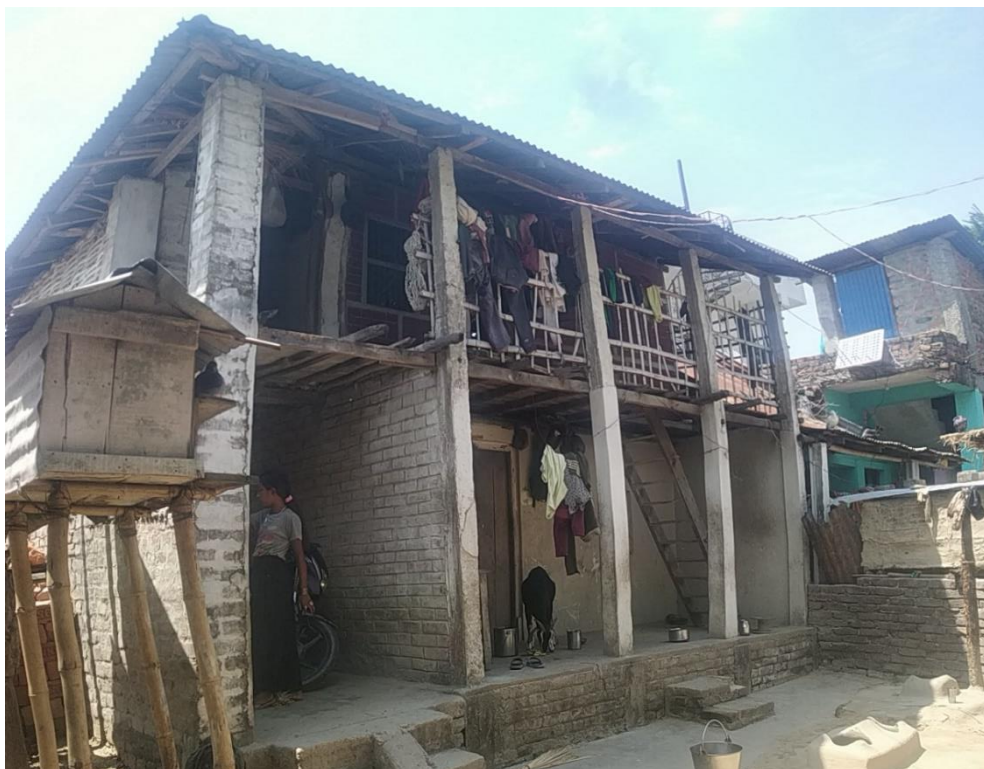
Figure 119: Addition of pillar and concrete block in old mud structure; Residence of Mr. Ram Kumar Chaudhary (School Teacher)
