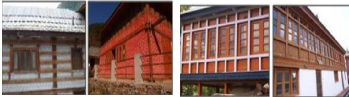
Figure 51: Absence of Kath Kuni style with use of concrete blocks
