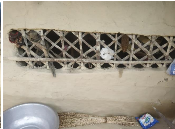
Figure 33: Criss-cross pattern of window opening without frame and shutter
