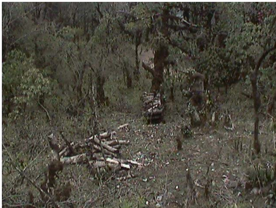
Figure 18. Dobato-Kalpokhari Road Under Construction . First trees are cut then the road is dug. In the center of the photo is a woodpile, the lighter area behind this is the newly dug road. This road has been constructed without having been surveyed by the Ilam District Development Office.
