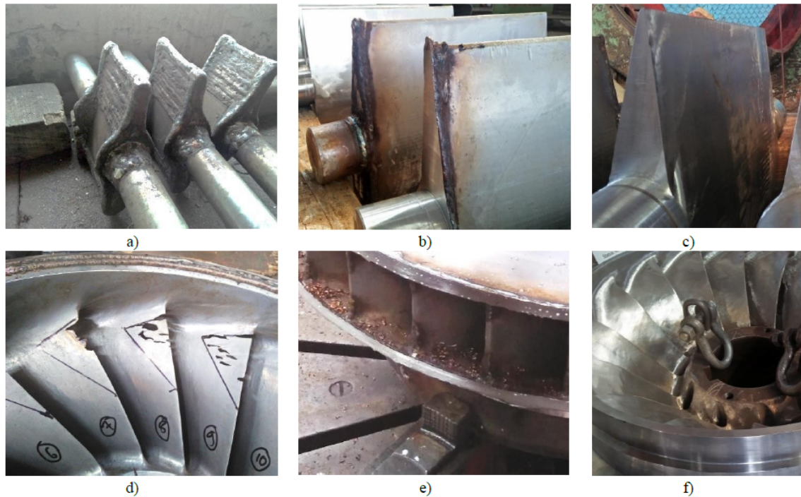
Figure 2.3: Different processes of repairing eroded GVs (a, b, c) and runner (d, e, f)
