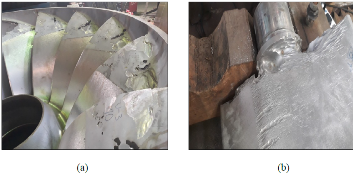
Figure 3.5: (a) Eroded runner blades (b) Eroded GV of Kaligandaki 'A' hydro-power plant
