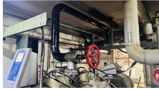
F. Refrigeration Pipelines
