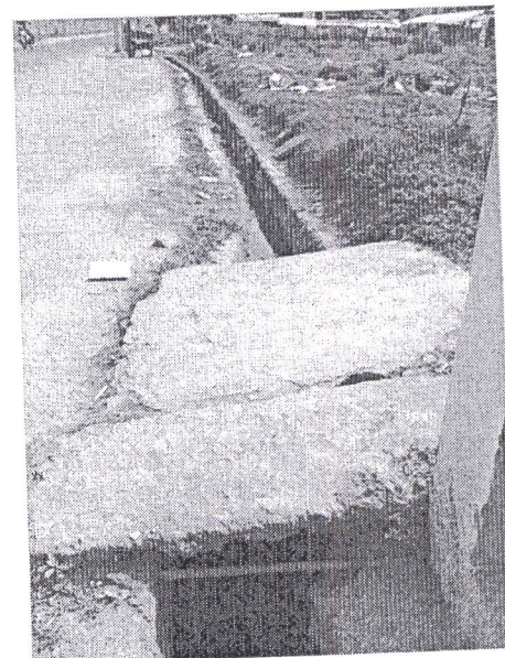
Figure 24 Open drain system in Saibu VDC
