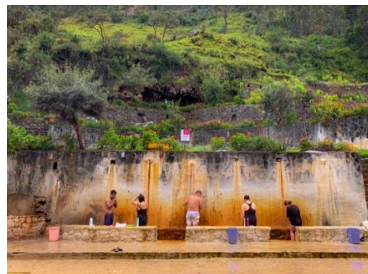
Figure 35 Shower walls bleached due to minerals present in the water
