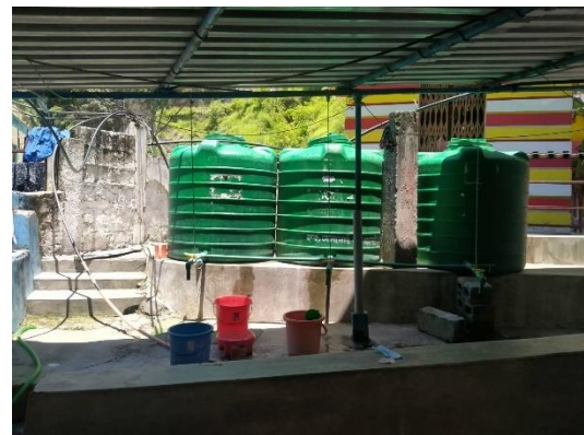
Figure 64 Water Tank (2000L tank-2, 1000L tank-3)
