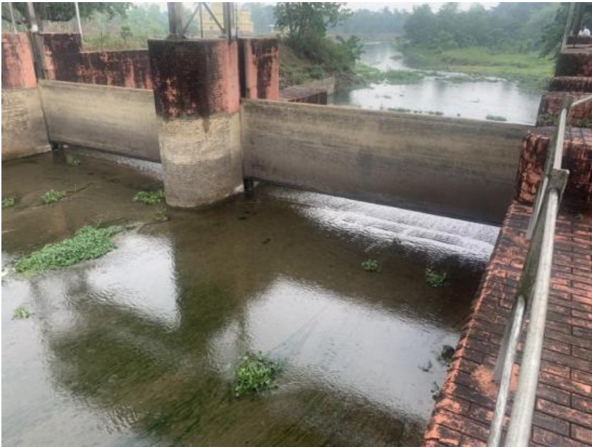
Water flow inside head works of Khageri river
