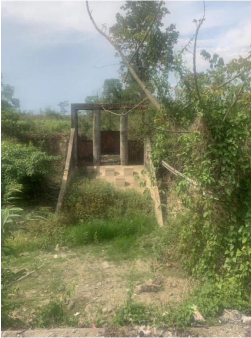
Current operation mechanism of irrigation sluice gate
