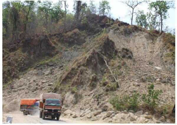
Figure: Reactivated landslide at the road section near Babai valley.
