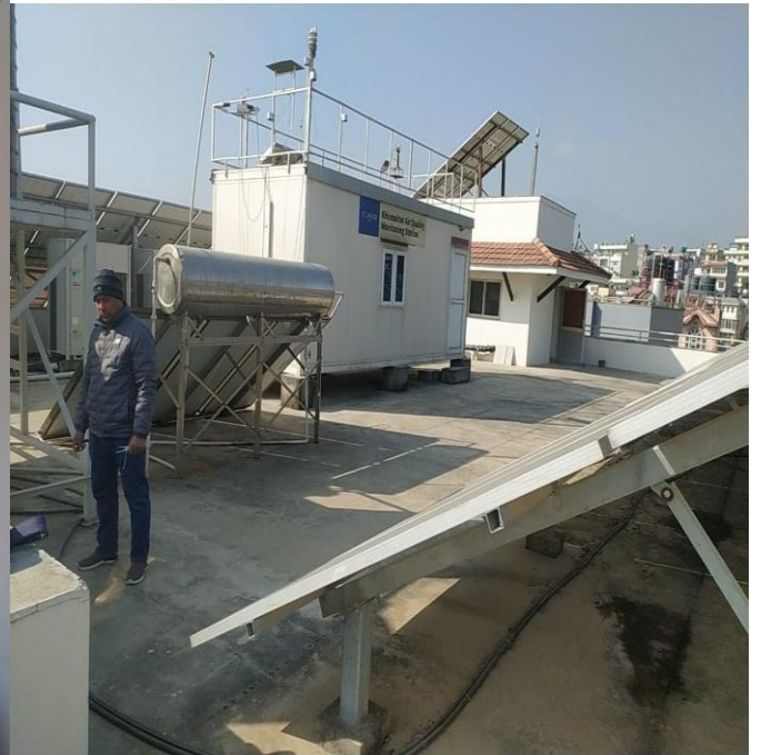
Figure 16 Concrete Roof with solar Panels
