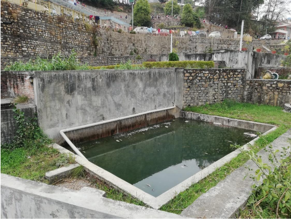
Figure 0.7: Vertical Flow Constructed Wetland
