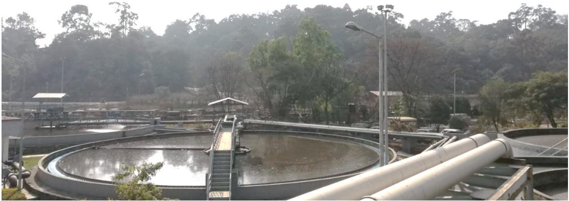
Figure 0.2: Secondary Sedimentation tank
