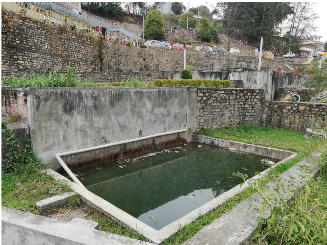
Figure 5.1: Aeration using tubes with holes to increase the Dissolved Oxygen in the Treated Water
