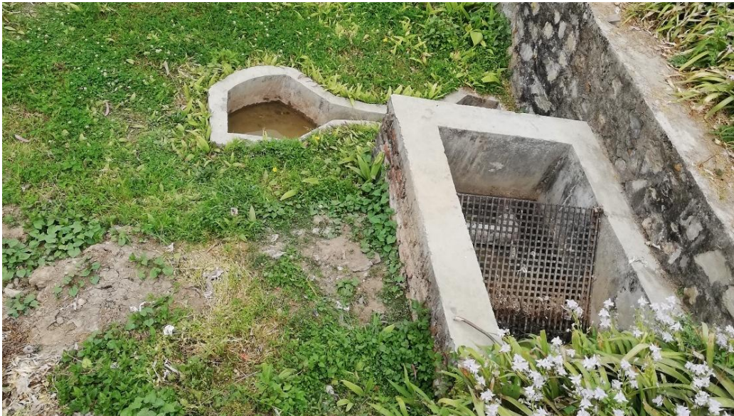
Figure 0.4: Screen Chamber and Cyclone at CW at Dhulikhel
