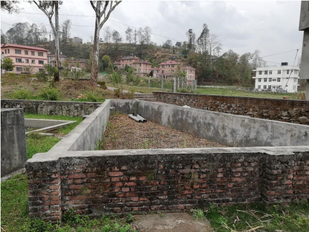
Figure 0.8: Sludge drying bed
