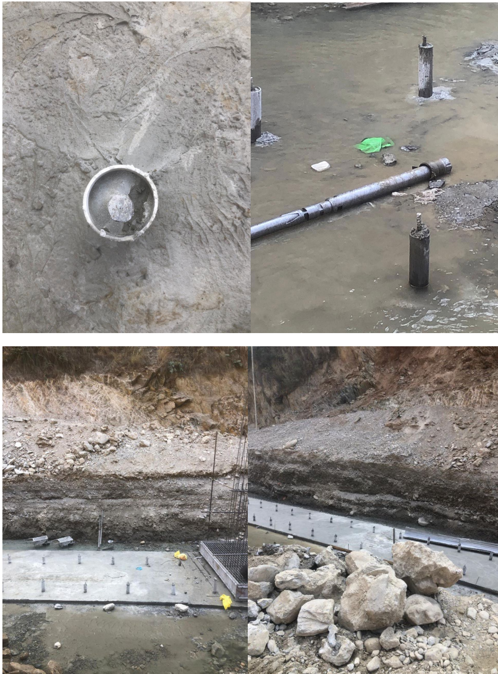
Figure: Photos of the case study site of cantiliver wall supported by micropiles. Photos were taken from the roshi section of the BP Highway, Kavrepalachok. Construction was carried out under the supervision of the Bhaktpur Road Division Office.
